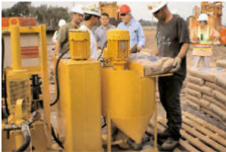
High Pressure Grout Plant
